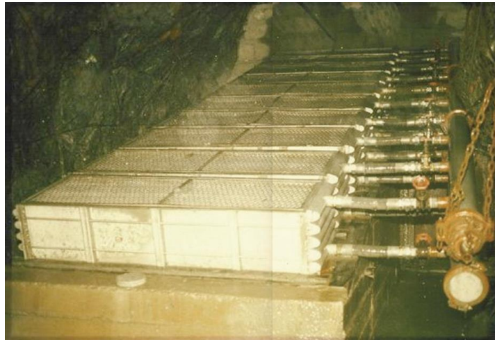
Figure 3: A closed-circuit cooling-coil heat exchanger bank (Mackay, et al., 2010)
