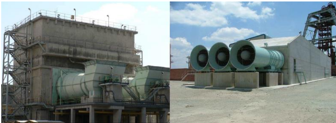
Figure 2: A vertical fill-packed tower BAC and a multi-stage horizontal spray chamber BAC (Roman, Glehn, & Marx, 2013)
