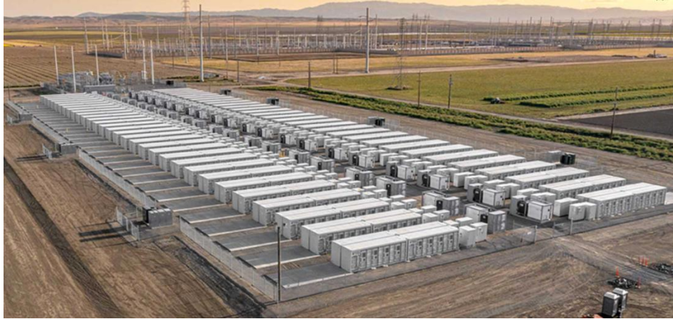
Figure 1.1 Project, named Fifth Standard, is RWE's largest U.S. storage facility to date, at 137 megawatts (MW), and includes a 150-MW solar PV array expected to be complete in August. When fully energized, the facility, located in Fresno County, will have the capacity to power more than 26,000 homes ( ref.11)
