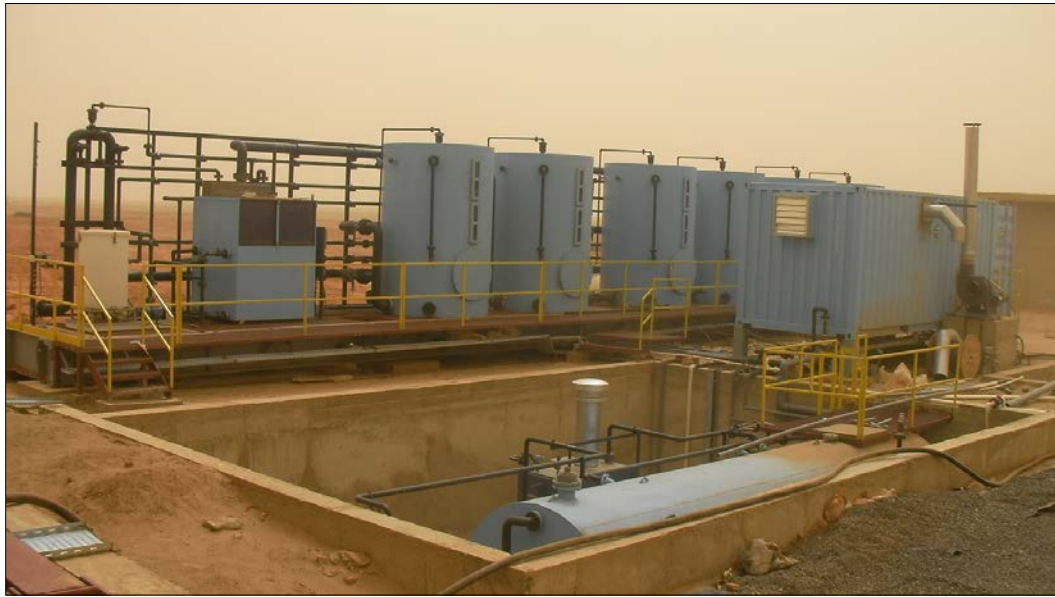
Figure 12. Modular Carbon in Column Process (CIC) Plant
