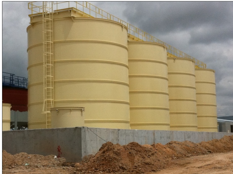
Figure 11. Agitated Leach Tanks in a Merrill-Crowe Plant
