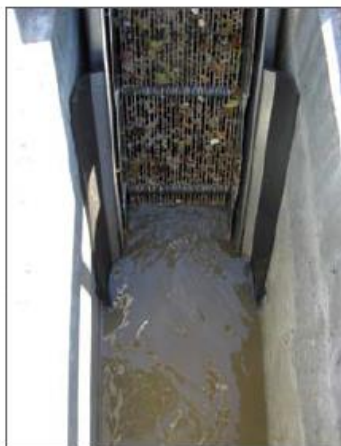
Screen in channel with neoprene seals.
