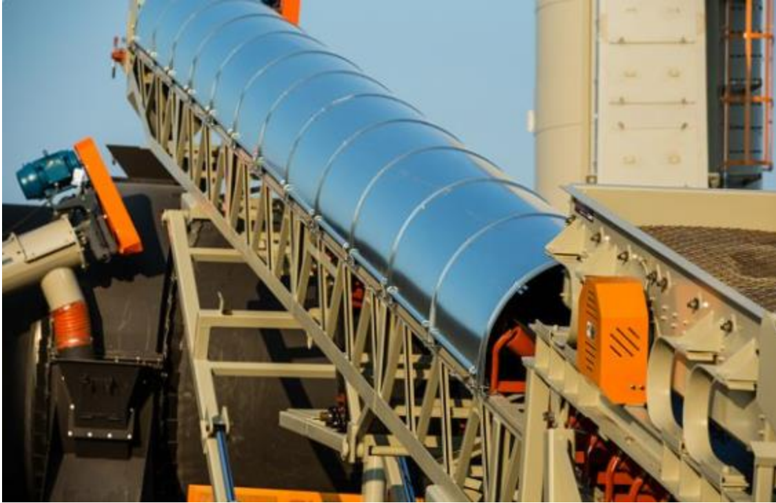
Figure 9. Conveyor Belt with Windshield Covering[8].
