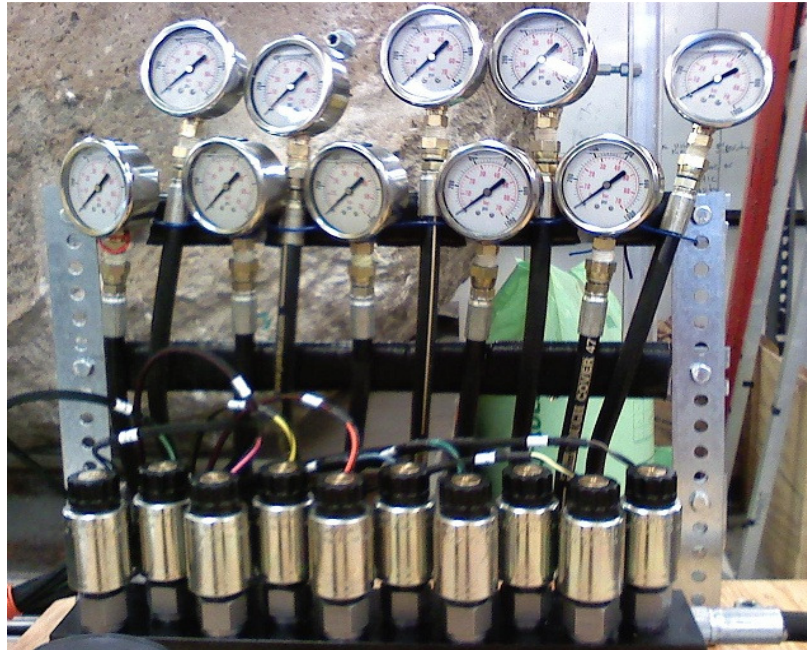
Figure 22: Electro-hydraulic valve bank
