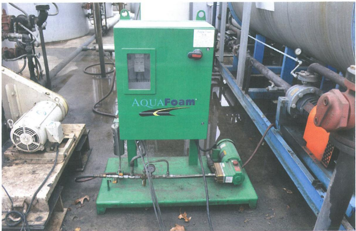
Figure 6 AquaFoam Metering Skid.
