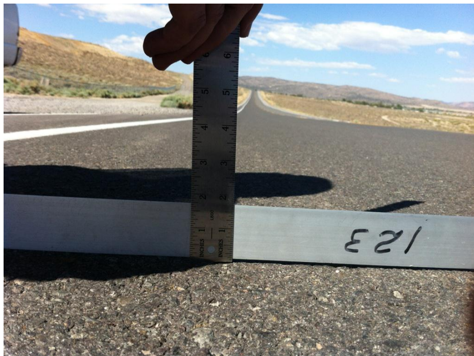
Figure 36 Maximum Rutting Depth of 1/16 Inches Measured (July 17, 2012).
