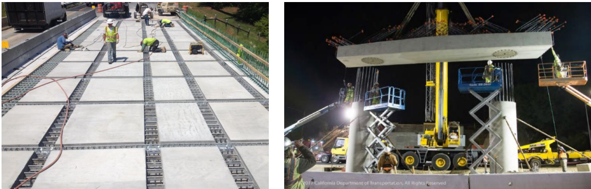
Figure 1. UHPC applications: (a) Precast deck panels with transverse and longitudinal joints [16], (b) Precast column and drop bent cap for Laurel Street Overcrossing project in California, USA (courtesy of Dorie Mellon)
