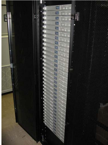
Figure 4.3: One rack of compute nodes in the UNR Research Grid [7]
